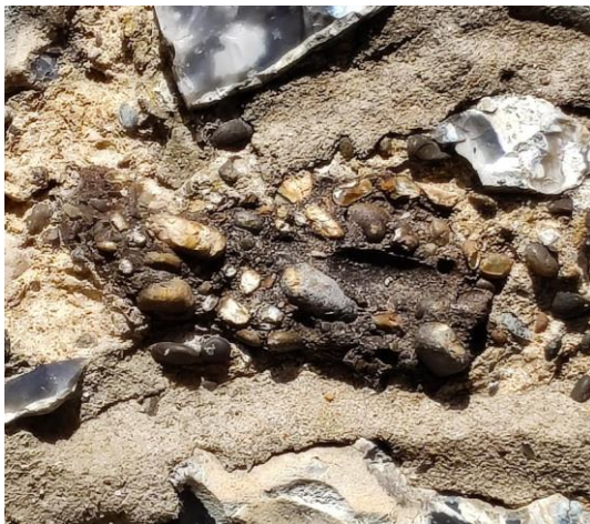
Figure 10: Puddingstone with iron stained cement.
