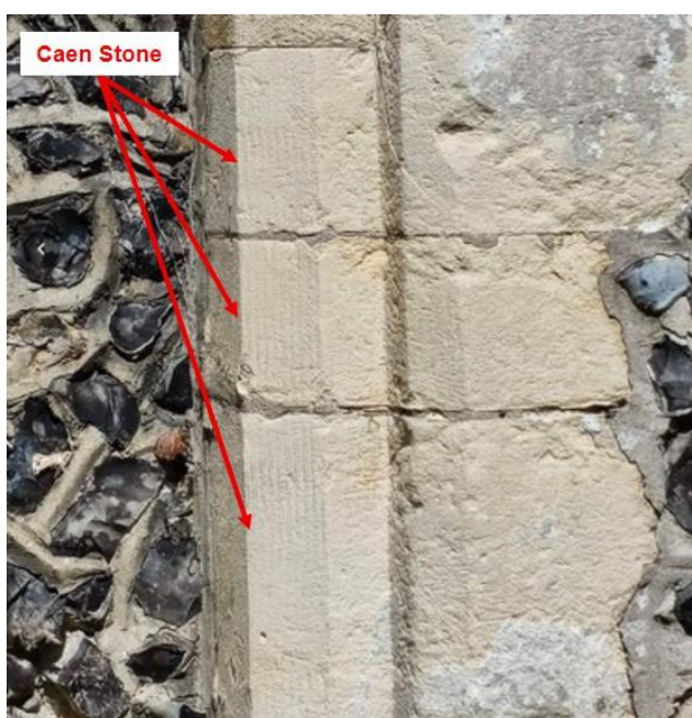
Figure 15: Caen Stone in south wall arch.
