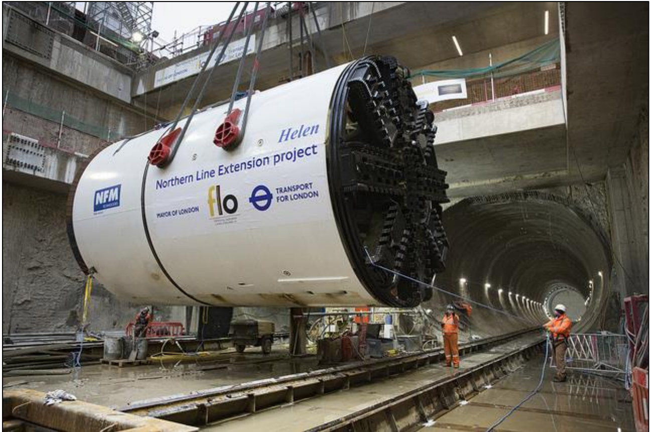
Figure 6: “Helen”, one of the two TBMs used in the Northern Line Extension. (Image: Londonist.com)
