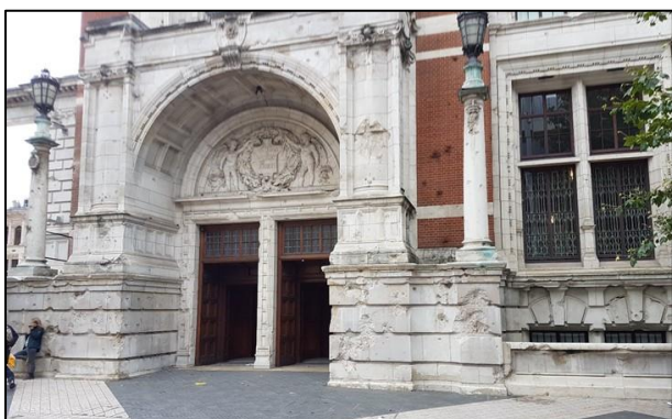
Figure 1: Bomb damage on the V & A Museum on Exhibition Road, South Kensington. Similar damage can be seen on the NHM Earth Galleries entrance on the other side of Exhibition Road.
