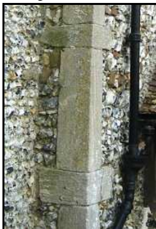
Fig. 3: A long and short quoin created in Barnack Stone in the mainly flint church of Strethall, Essex; note horiz & vert bedding.
