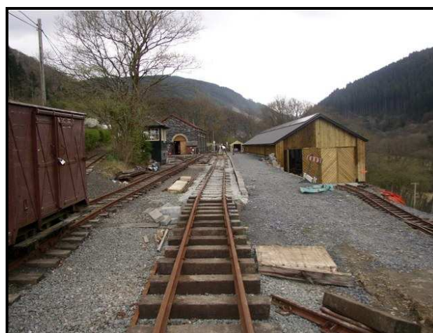
Fig. 2. Similar viewpoint to Fig. 1, Main Engineering Base in April 2009, showing engine shed (in distance Left) and new carriage shed (Right).
