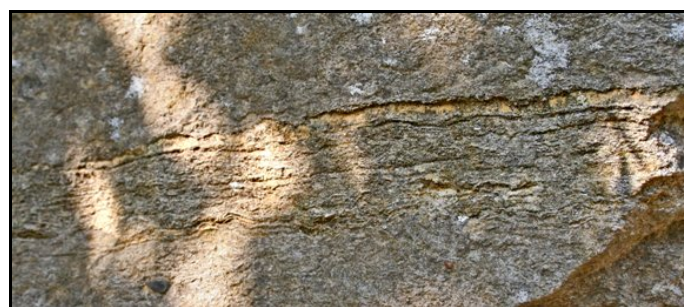
Evidence of algae
